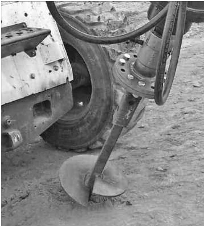
A skidsteer with a torque motor attachment is used to install the Helical Ground Anchor at the prescribed angle and depth for bracing.
